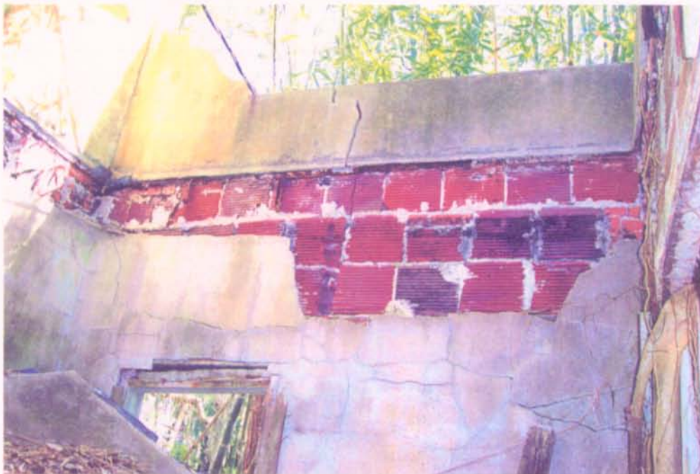
Photograph 6: DETAIL OF COLLAPSED ROOF OF LAUNDRY ROOM SHOWING PARAPET ABOVE ROOF, FLASHING DETAILS, ROOF RAFTER LINE AND ADJACENT STUCCO.
