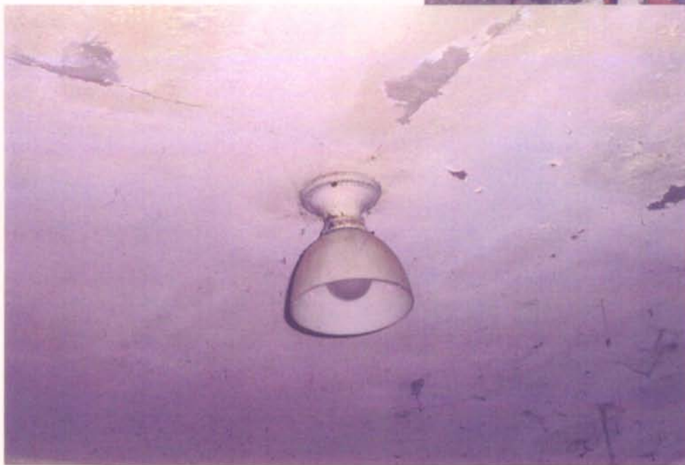
Photograph 20: DETAIL OF TYPICAL ORIGINAL ROOM LIGHT FIXTURE.
