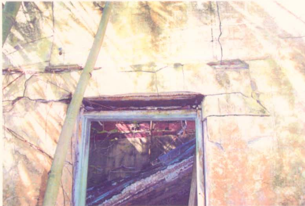
Photograph 4: DETAIL OF PARTIAL EAST ELEVATION WITH DOOR TO LAUNDRY SHOWING DETERIORATED STUCCO AND METAL LINTEL OVER DOOR.
