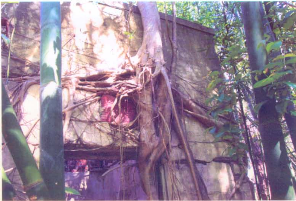
Photograph 3: DETAIL OF PARTIAL SOUTH ELEVATION SHOWING TREE GROWING FROM WALL WITH ROOTS EXTENDING TO SIDES AND DOWN.
