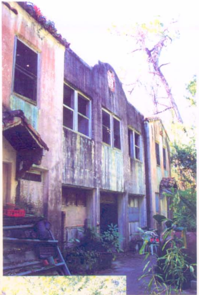
Photograph 1: NORTH ELEVATION SHOWING GENERAL CONDITION OF BUILDING NOTE STAINED STUCCO WALL FINISH AND DETERIORATED WINDOWS.
