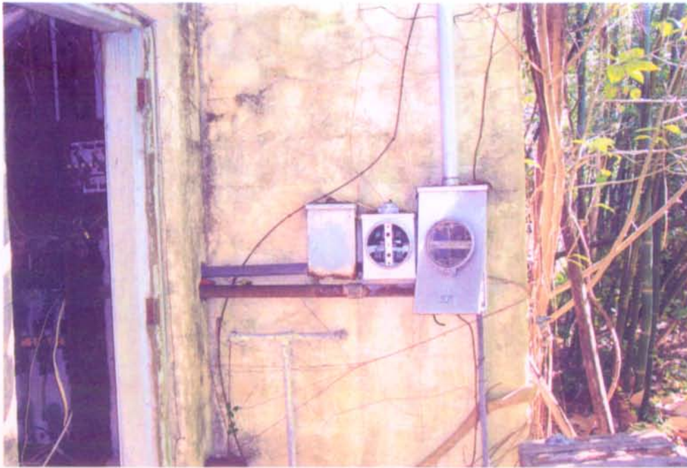
Photograph 5: DETAIL OF ELECTRICAL SERVICE ENTRY ON SOUTH ELEVATION.
