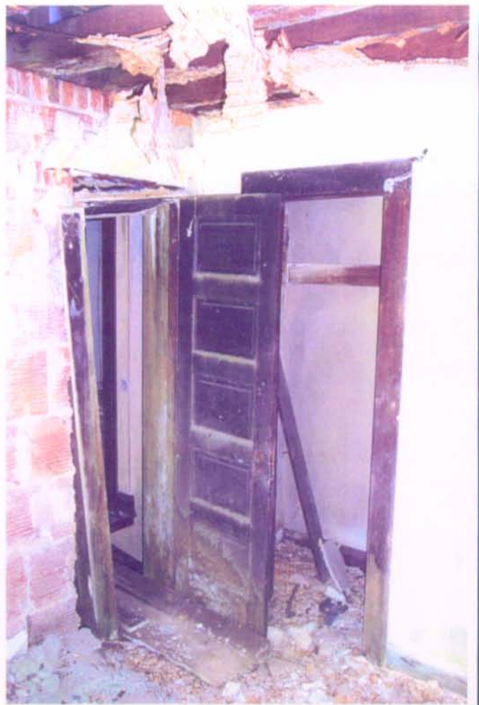
Photograph 11: INTERIOR ELEVATION OF DOOR AND CLOSET ON SECOND FLOOR SHOWING DETERIORATED CONDITION.
