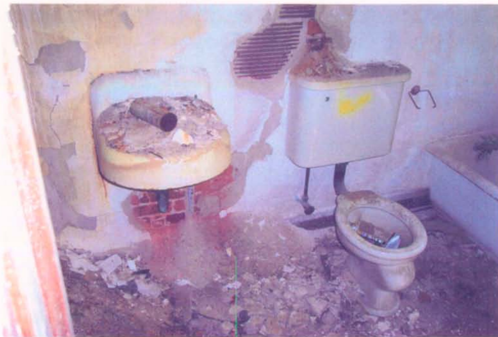
Photograph 18: DETAIL OF BATHROOM SHOWING FIXTURES AND GENERAL DETERIORATION.
