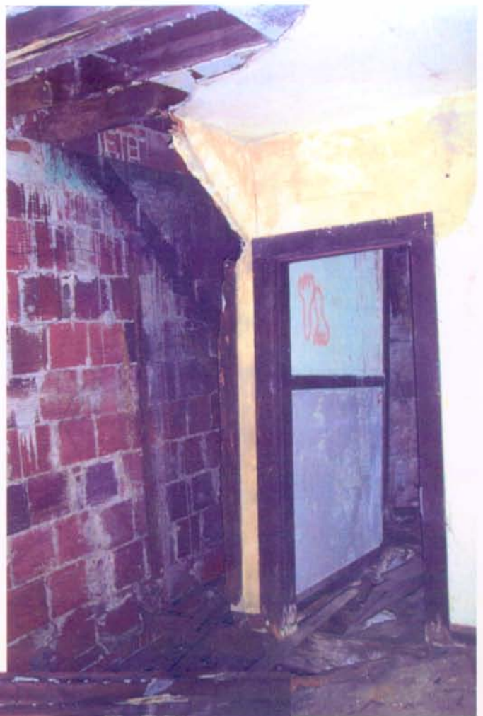
Photograph 7: DETAIL OF INTERIOR FIRST FLOOR SHOWING DOOR TO KITCHEN, DOOR TO CLOSET UNDER STAIR AND GENERAL DETERIORATED CONDITION.
