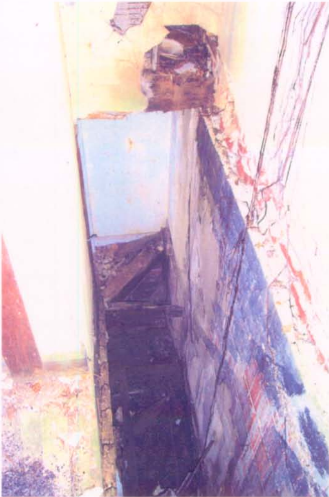
Photograph 12: VIEW FROM SECOND FLOOR LOOKING DOWN INTO STAIR WELL WITH MISSING STAIR.
